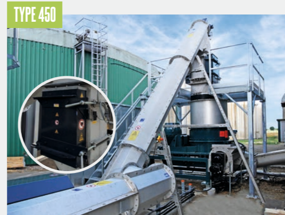
A two-part screw conveyor system consisting of a TYPE 450 horizontal and an inclined screw conveyor with magnetic separator transfers the substrate to a vertical shredder.
