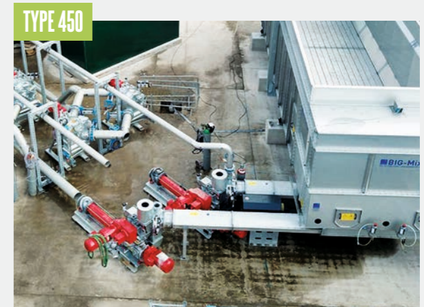
A feed system with two connected TYPE 450 screw conveyors simultaneously feeds two external liquid feed systems.
