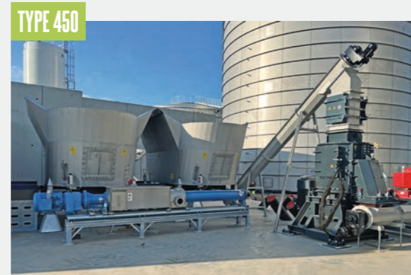
Two independent feed systems feed two liquid feed systems. One of them feeds into a vertical shredder via a two-part TYPE 450 screw conveyor system with magnetic separator. It is then transported to an external liquid feed system by a TYPE 450 flex transfer. The other is equipped with a TYP 450 horizontal screw conveyor with flexible transfer that conveys into an external liquid feed system.
