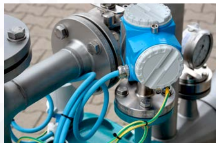
Electronic leak monitor
