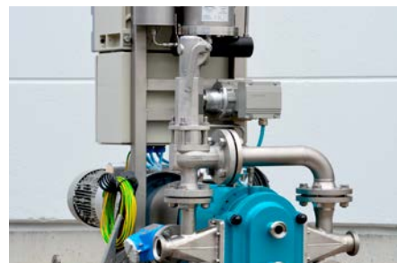
Overpressure protection by bypass with safety valve
